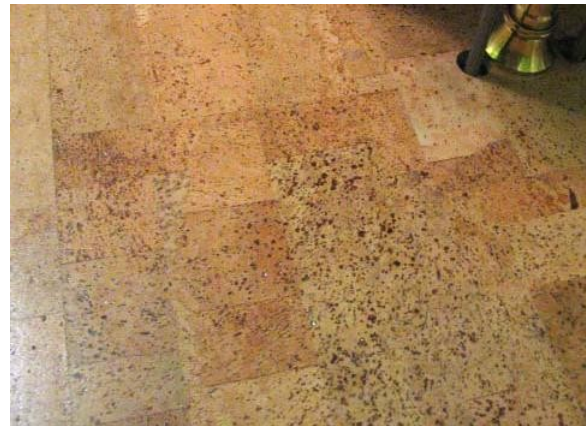
Cork flooring is very "Green", relatively inexpensive, very water resistant and absolutely beautiful as well as a treat to walk on.
